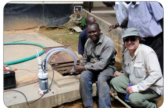
Staff member Doug Lark installing a M-100 at St. Luke's Mission Hospital in Kaloleni, Kenya July 2012.
