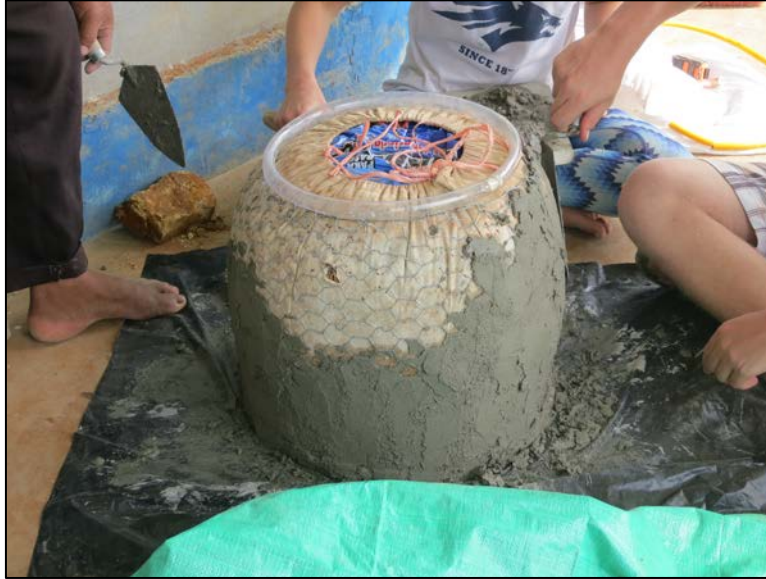
Enrique, Austin, and Brittany add the first coat of cement to the 12-gallon tank.
